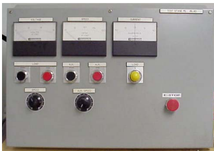
One of several load control stations at our facility
