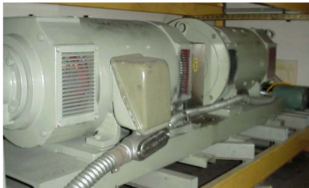
One of 9 Coupled AC/DC Motors/Generator sets for testing Drives under loaded conditions ( many small repair shops cannot verify drive operation under loaded conditions as it requires considerable investment )
